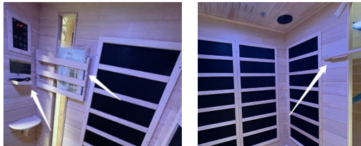
(Figure C: Accessories installed inside the sauna)
